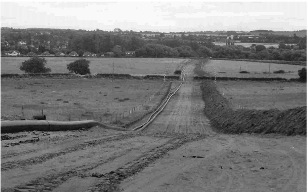
New pipe line from Palmers Hill looking back to old sewage works
