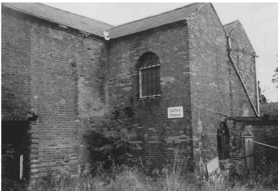
Machinery House at Wassell Grove Farm housing animal food preparation machines and driven originally by a steam engine
